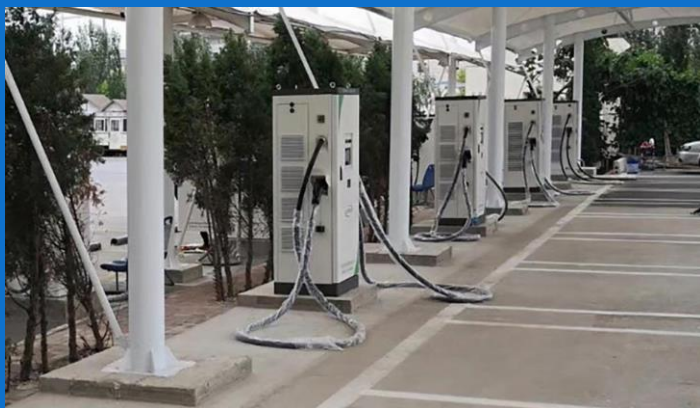
Jiangsu State Grid Project
