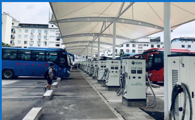
Shanxi State Grid Project
