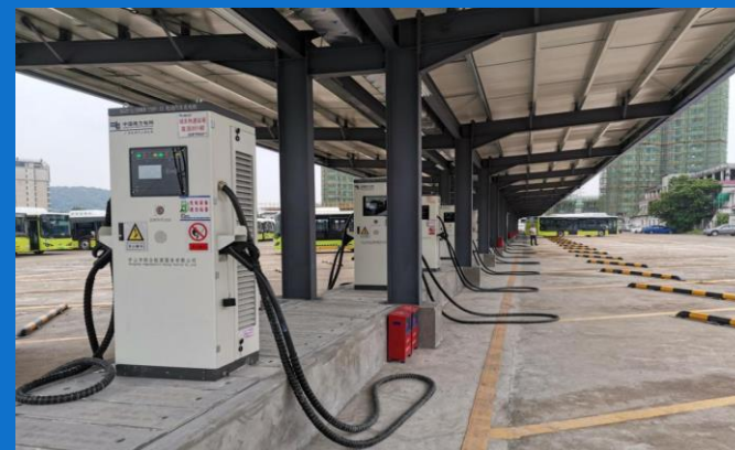
Tianjin State Grid Project
